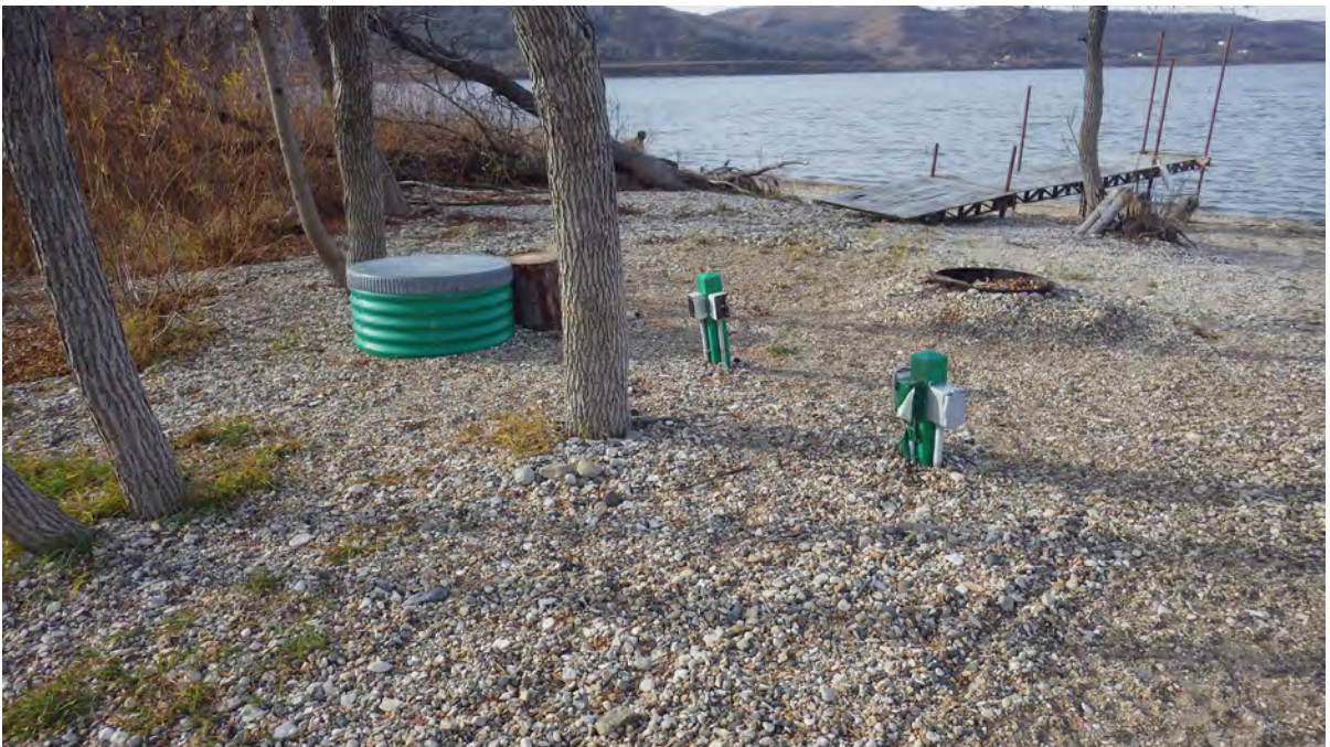
Figure 14: Electrical infrastructure near the cleared area
