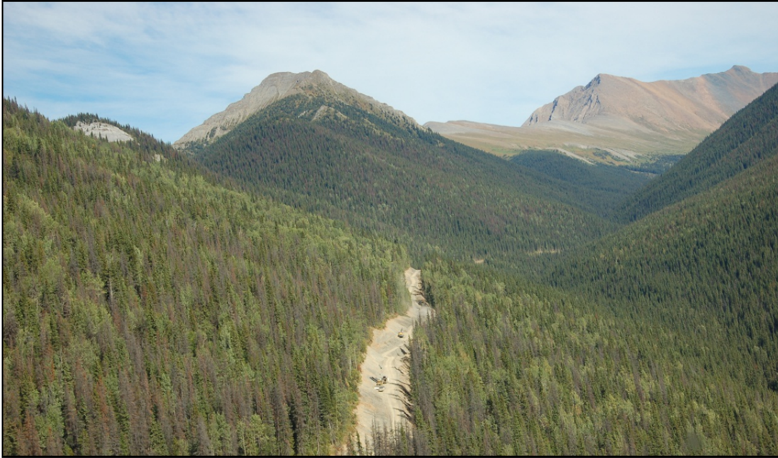
Photograph 3 – the site access road currently under construction. The road, constructed to support exploration activities, links into the existing forestry road network.
