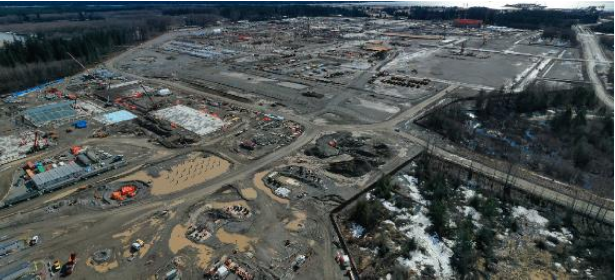
PHOTO 5: LNG FACILITY – DRONE SHOT (MARCH 2021)
